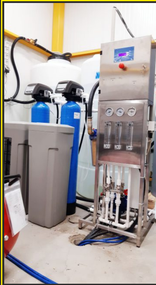
WATER SOFTENING & REVERSE OSMOSIS SYSTEM
